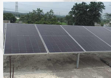
Ensuring a sustainable source of electricity through solar panels at Zilla Parishad Prathamik School, Waghru, Jalna
